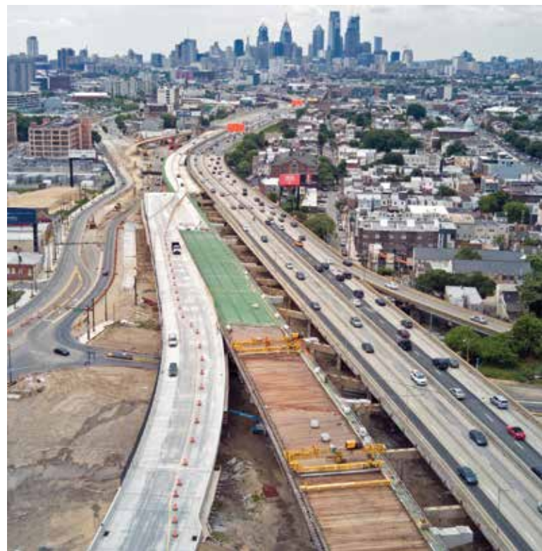
Northbound I-95 traffic exiting at Girard Avenue uses the new off-ramp to Richmond Street as deck construction progresses south toward Palmer Street. (Note the burlap covering recently poured concrete at the bottom of the photo and the as-yet unpaved segment with green re-bars in place.) Photo: James J. Anderson Construction
