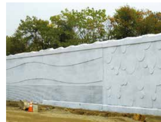
Thematic form liner treatment on a retaining wall along relocated Richmond Street near the Girard Avenue Interchange
