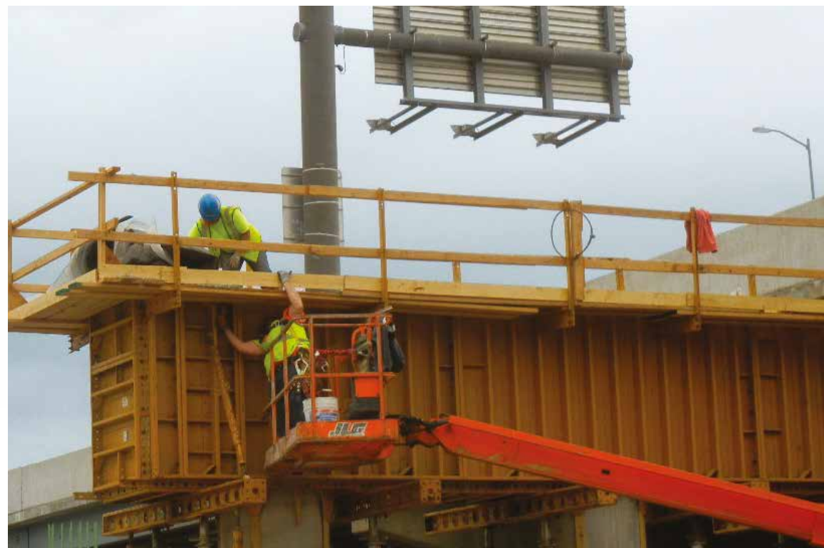
Workers build forms for a pier cap for widening southbound I-95 approaching Cottman Avenue.
