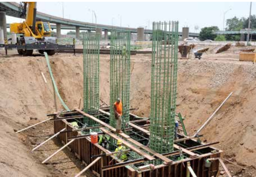
Left: Workers construct piers that will support widened and improved ramps along the southbound lanes of I-95 at the Betsy Ross Bridge/Aramingo Avenue Interchange.
